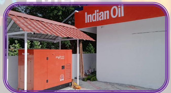
Diesel Gensets from Mahindra Powerol
